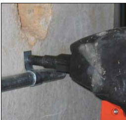
12HSMP034 clip assembly used to secure conduit
