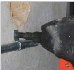
12HSMP034 clip assembly used to secure conduit
